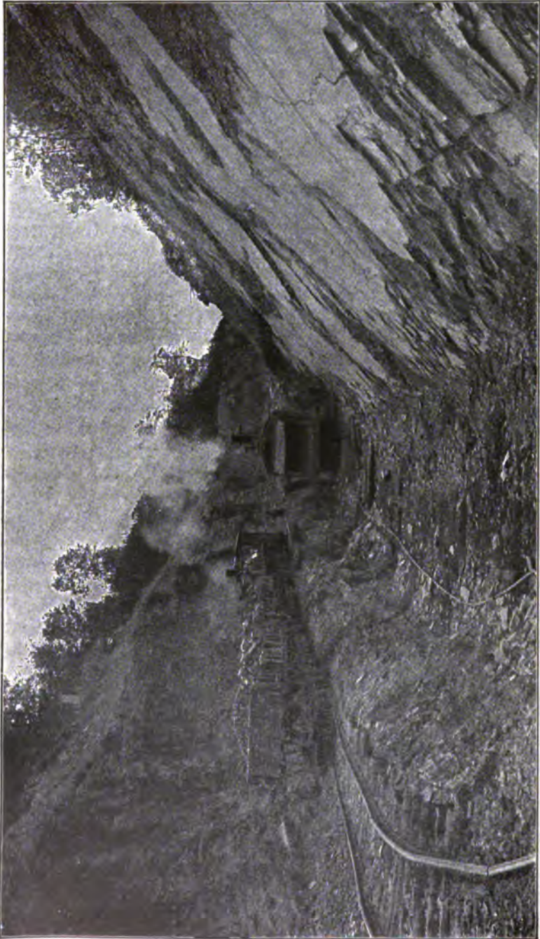
PLATE 109.—Contract 47. Excavation of Freer Cut in Sliding Hudson River Shale. Slope on right was very troublesome, large slabs breaking off and sliding, on "slickensided," planes into cut.
